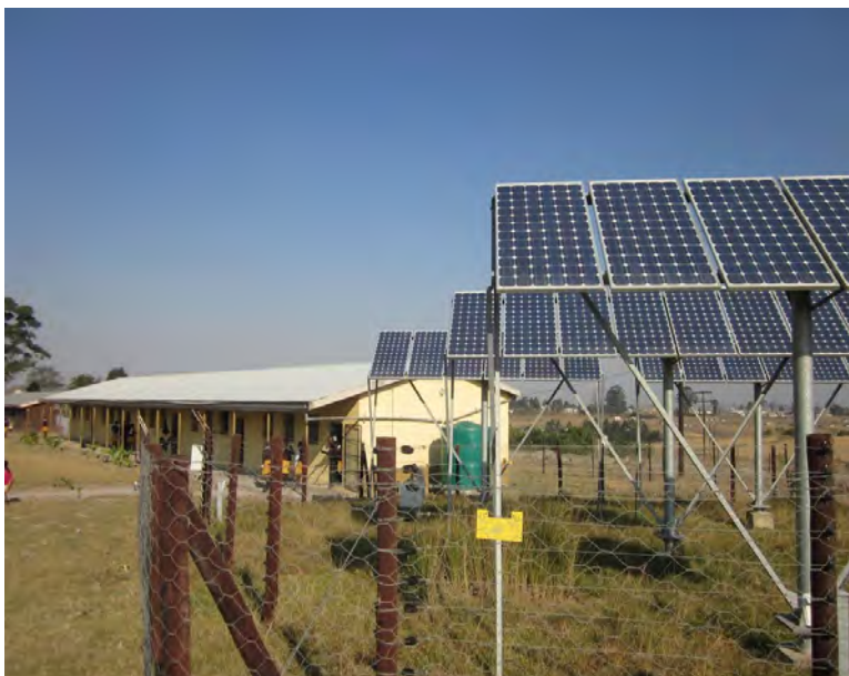
Providing renewable energy to a rural school.
