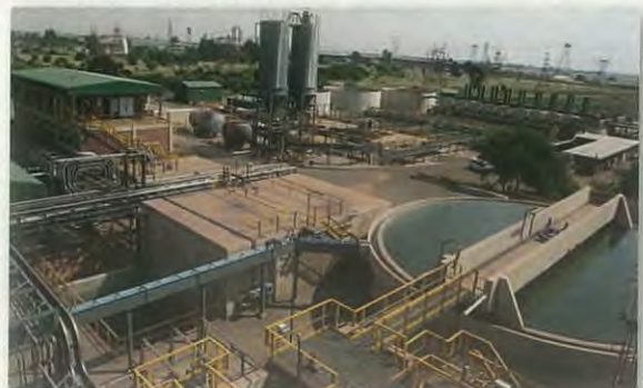
Main Treatment Plant at Mittal Steel South Africa, Vanderbijlpark
