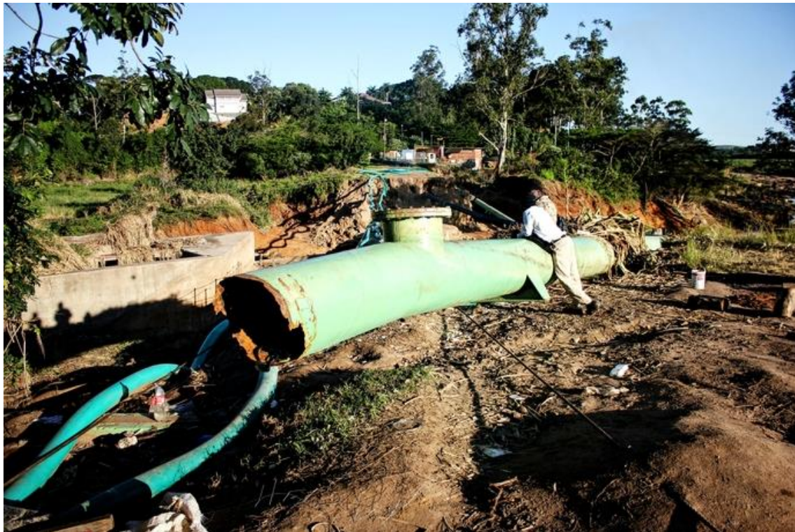
Damage to infrastructure. Photo: RLS Southern Africa
