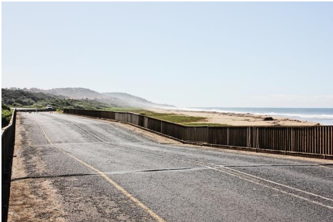
Road damaged by floods in Durban. Photo: RLS Southern Africa
