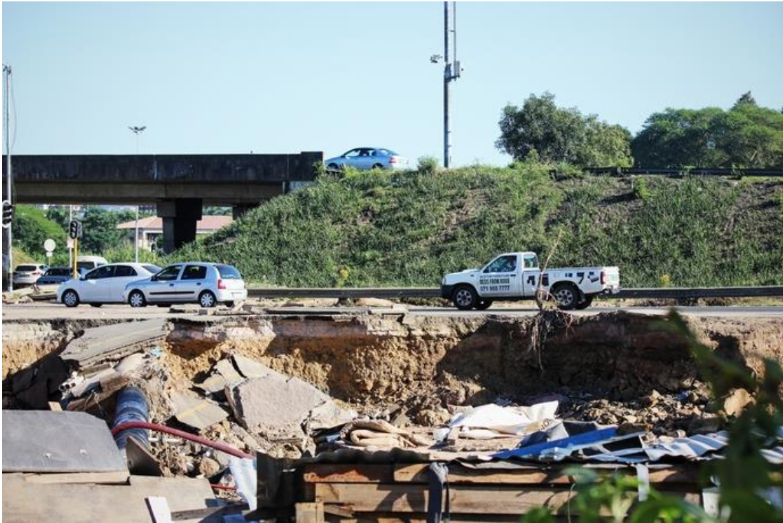
Climate change already causing unprecedented damage to public infrastructure. Photo: RLS Southern Africa
