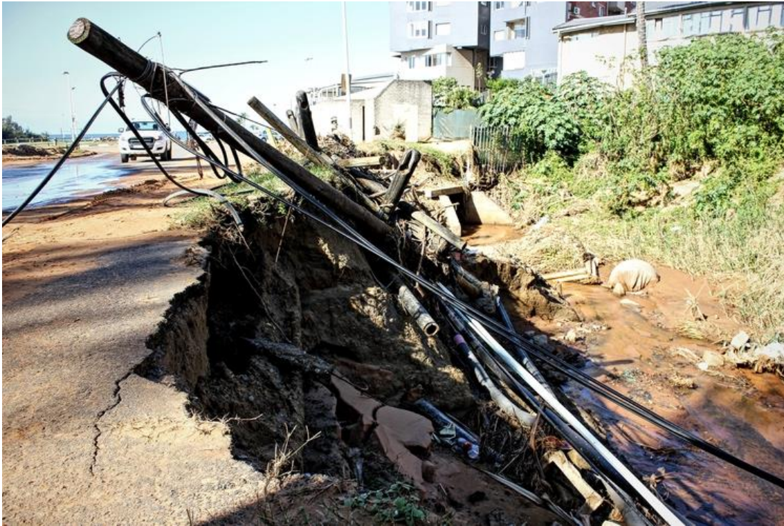
Power lines downed by floods. Photo: RLS Southern Africa
