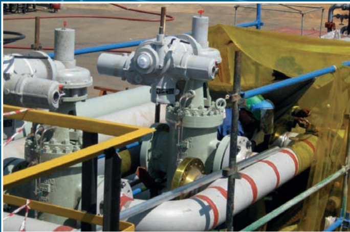
New Multi-Product Pipeline (NMPP)
